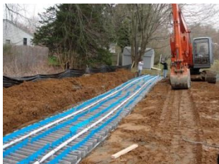
Installations of GeoU
